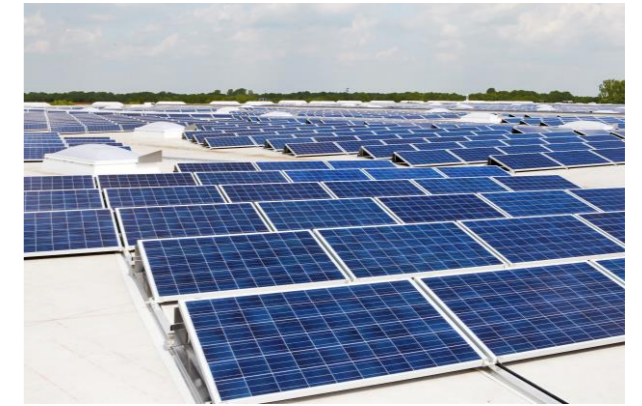
Figure 49 – PV Panels placed at 35 deg
